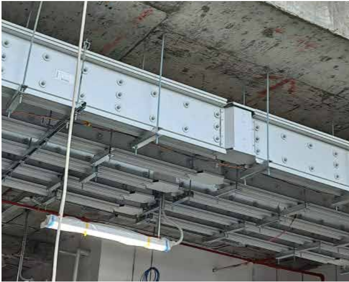
Example of Bahra busbar system
